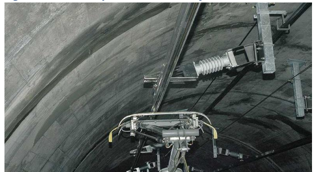
Figure 2. Furrer+Frey contact bar electrification
